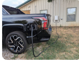
Detached building. Subpanel and charger at a shop, away from the house.
