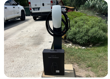
No wall to mount on. Pedestal on a poured pad, right where the car sits.
